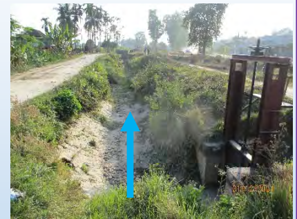
Parshall Flume is not installed (S-0)
