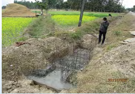
Construction of Field Outlet from TC-2 to Existing Field Channel (Model Site of S-17, T-2)
