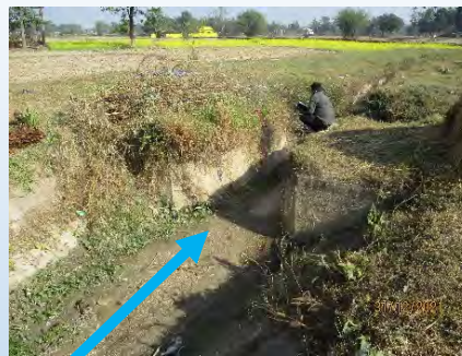
Parshall Flume is already installed (S-1)
