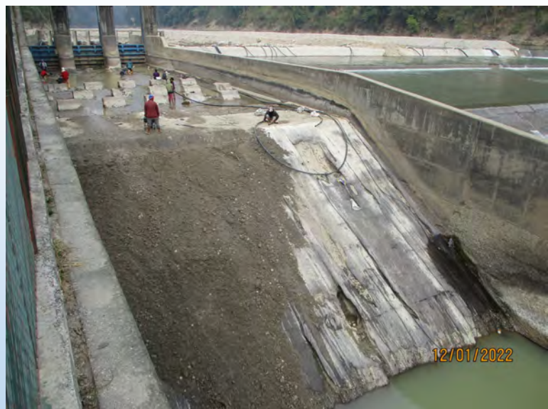
[Photo of Contractor's Work at Head Works] Rehabilitation of Undersluice of Kankai Headworks
